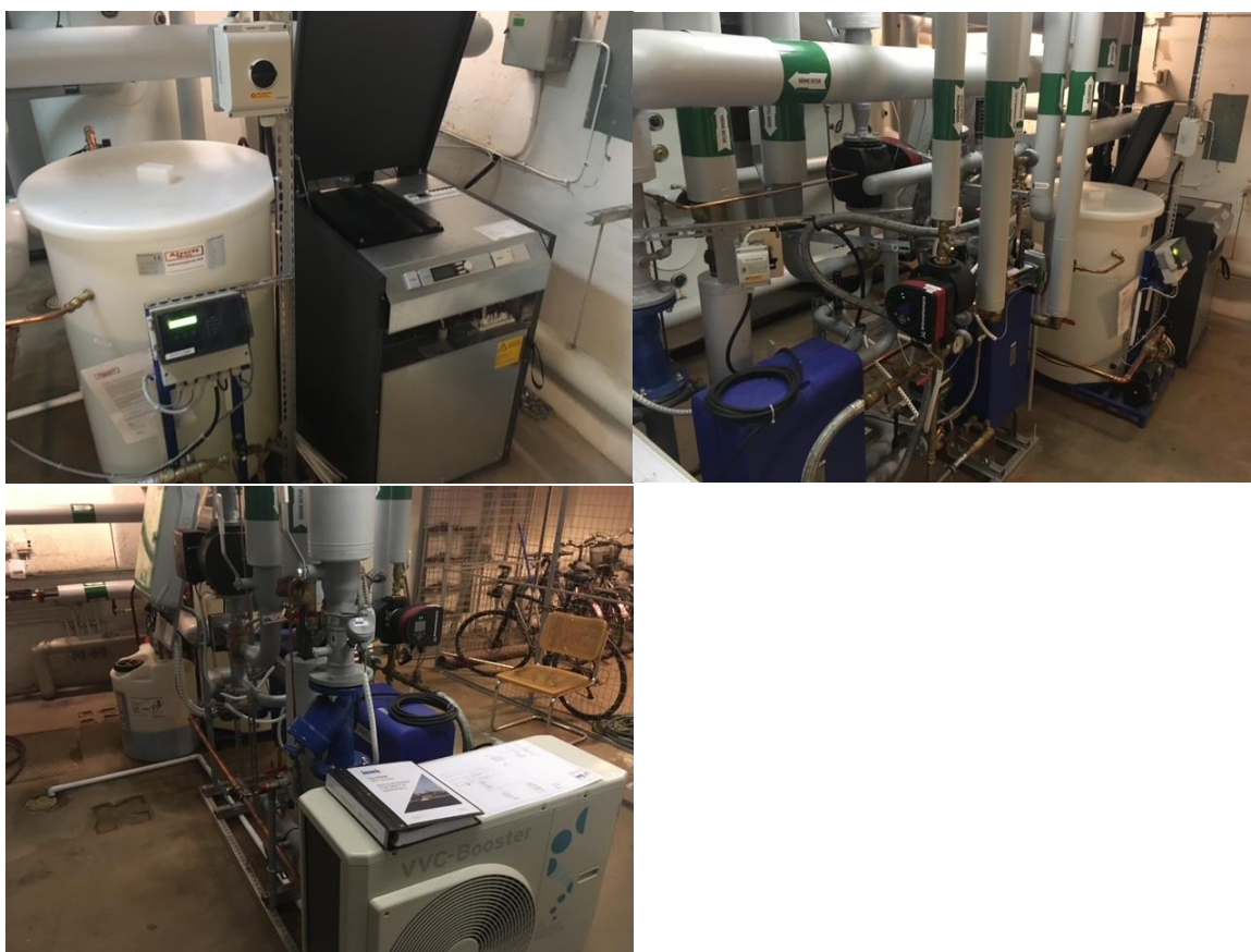
Nya installationer i undercentral.
